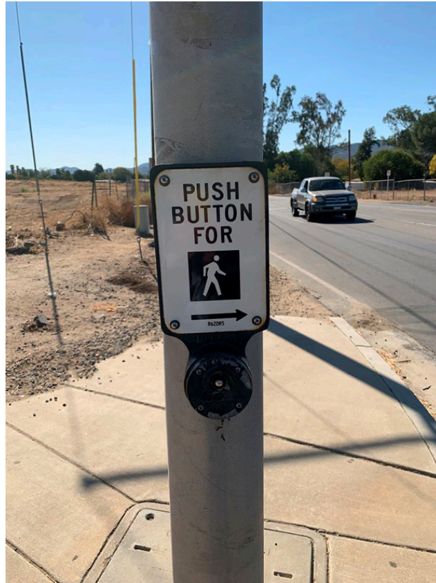
Figure 3.5: Non ADA-Compliant Pedestrian Push Buttons
