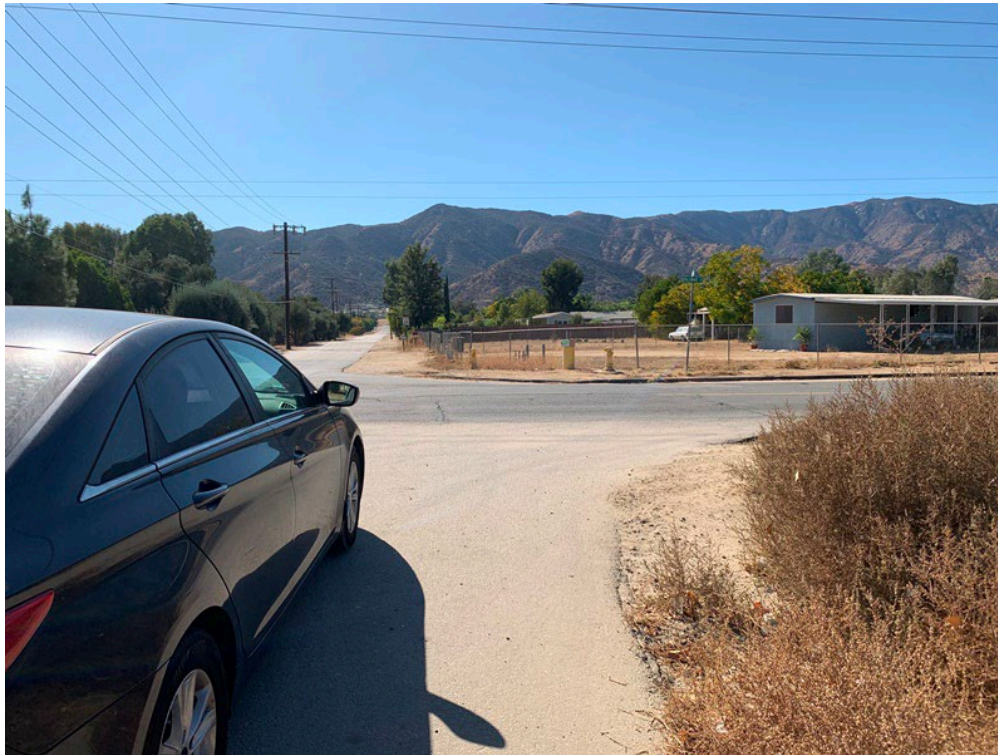
Figure 3.14: Missing Stop Sign and Pavement Markings on the Bryant Street North of Palomar Street
