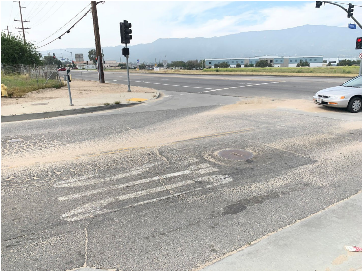
Figure 3.8: Non-Compliant STOP Pavement Marking Located at Mission Trail and Lemon Street
