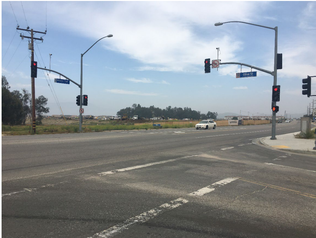
Figure 3.3: Faded Crosswalks at Mission Trail and Olive Street
